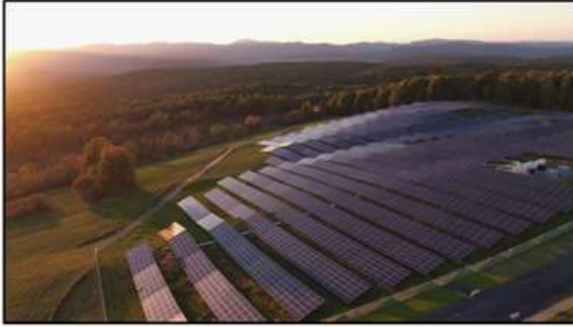
Large-scale ground-mounted solar array. Source: GZA GeoEnvironmental, Inc.
