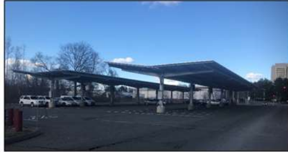
Canopy solar at a UMass Amherst parking lot. Source: GZA GeoEnvironmental, Inc.
