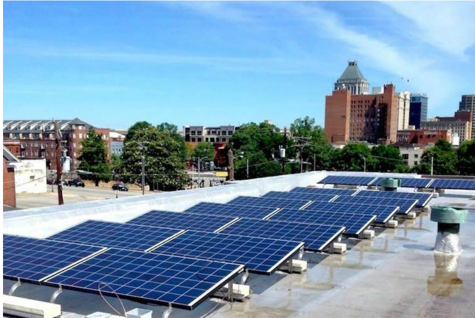
Figure 18. Rooftop Solar (Source: Inside Climate News)
